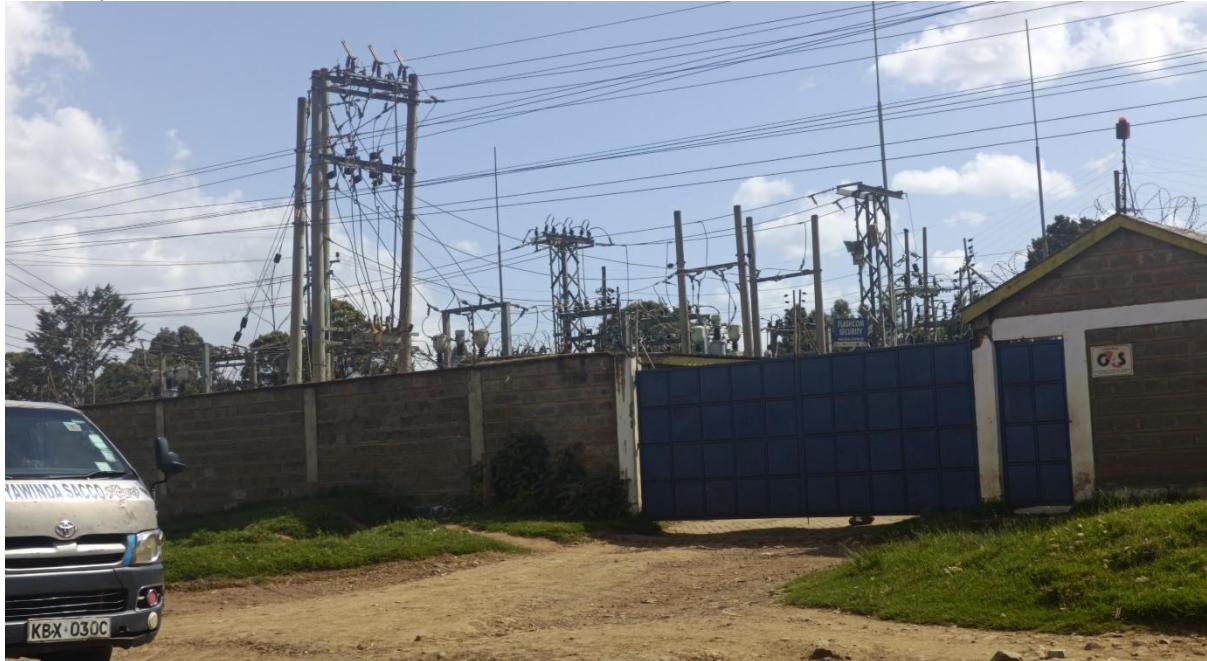
Plate 5: Nyahururu Power Substation
