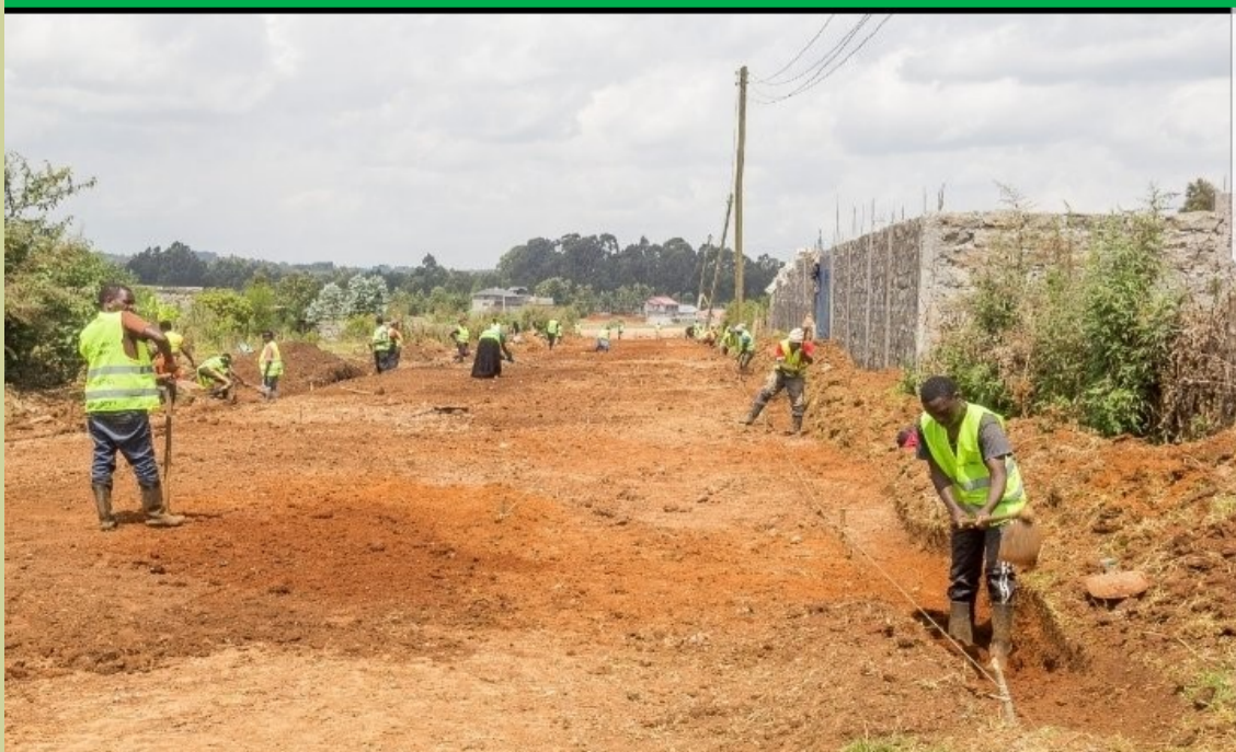
Youths rehabilitating road in Nyahururu, Igwamiti Ward under the civil works programme
