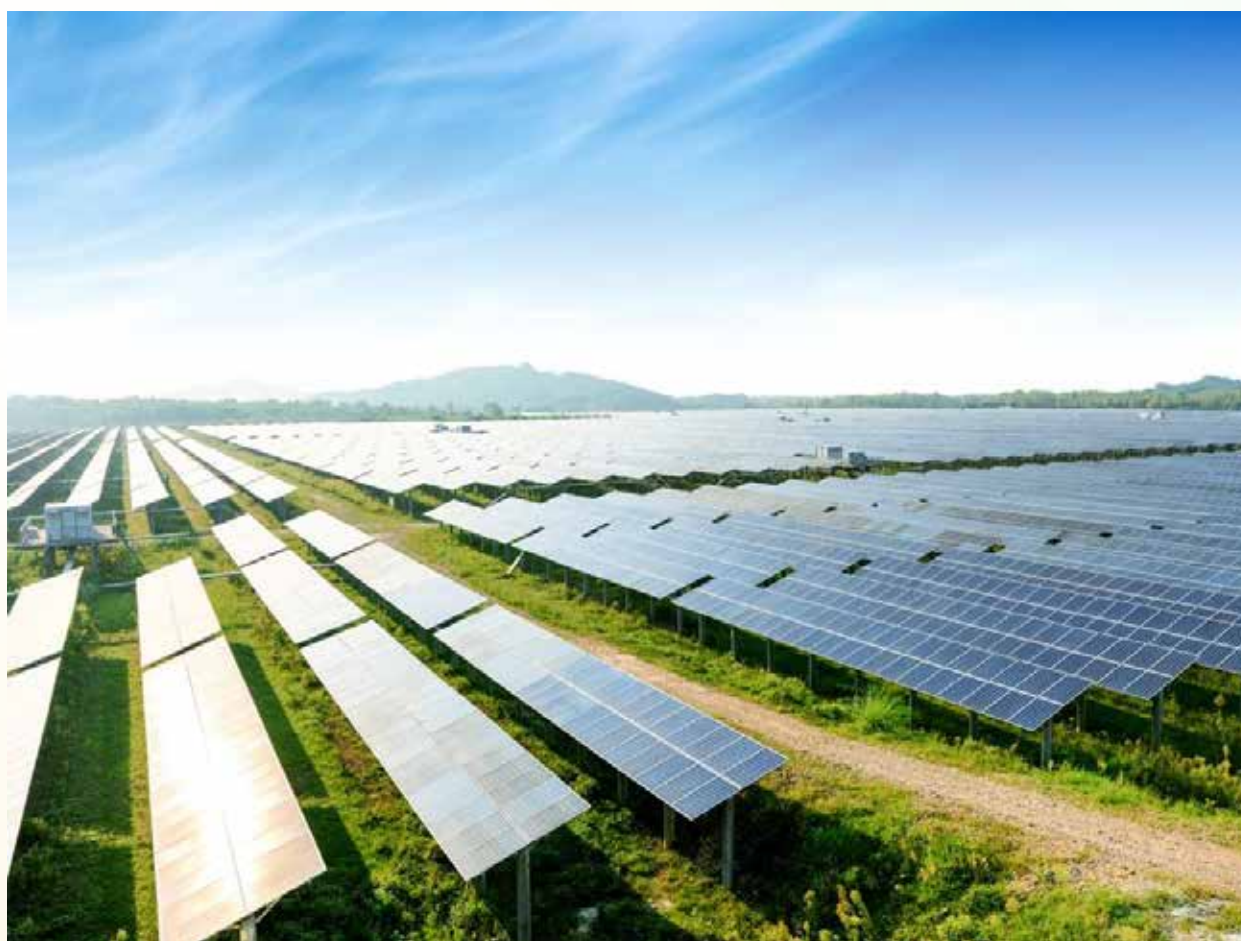
40- megawatt solar plant in Rumuruti
