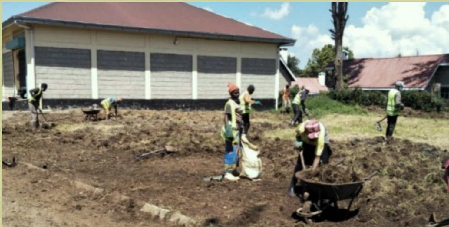
A section of the youths working under the Civil Works Programme in Nyahururu, Igwamiti Ward
