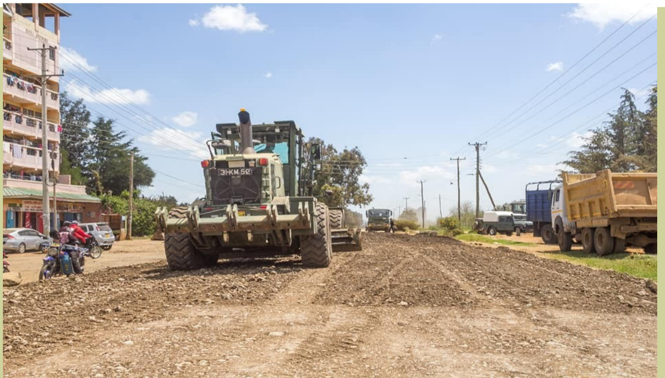
A brigade from BATUK working on a badly worn down section Laikipia Road in Nanyuki recently. The contractor working to restore the road is making slow progress, one month after the date of start of contract
