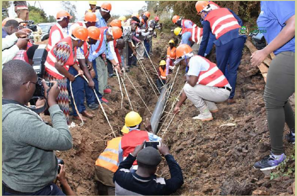
Governor Ndiritu Muriithi leads a team in laying pipes for the Solio Water project
