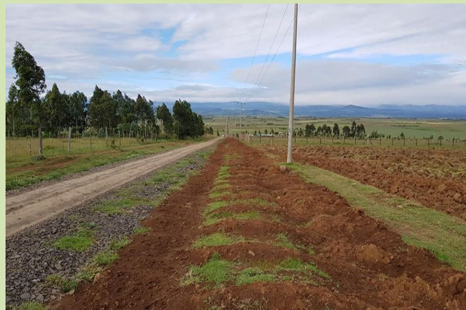
A section where the 34 km Solio water pipeline passes through
