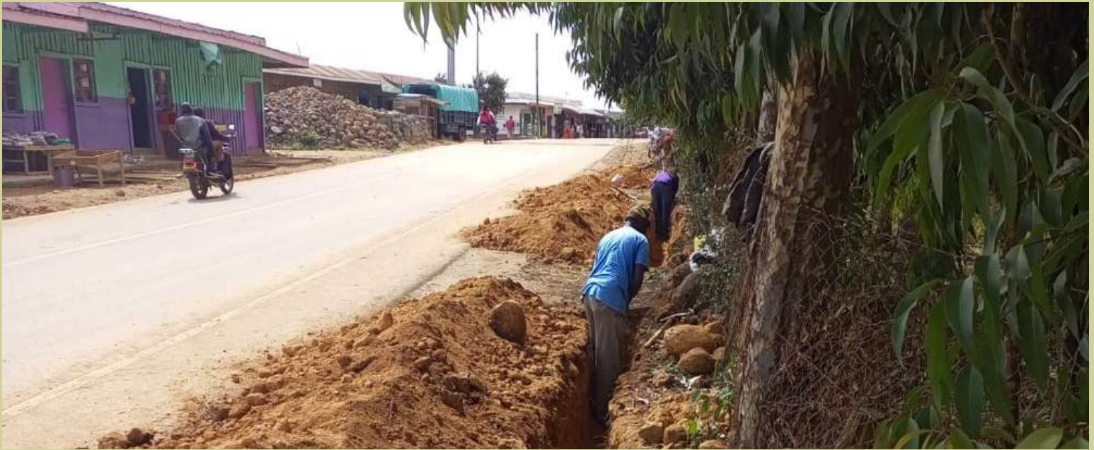
Digging of pipe trenches in Kinamba town Below: Offloading of pipes for Kinamba water project
