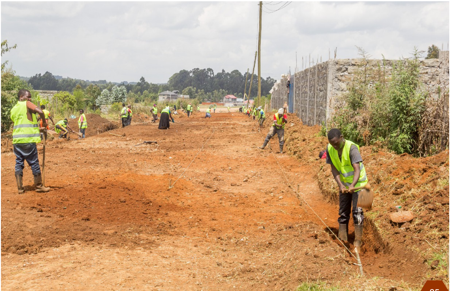
Youth working on a road in Nyahururu under the civil works programme of county government of Laikipia
