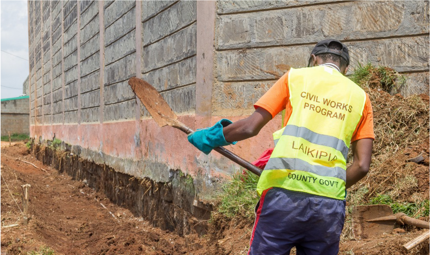
Youth working on a road in Nyahururu under the civil works programme of county government of Laikipia
