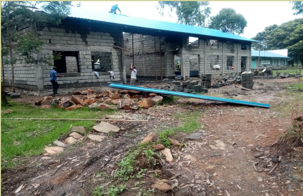
A motor vehicle workshop underway. At Nyahururu VTC It will be accessible to public once complete
