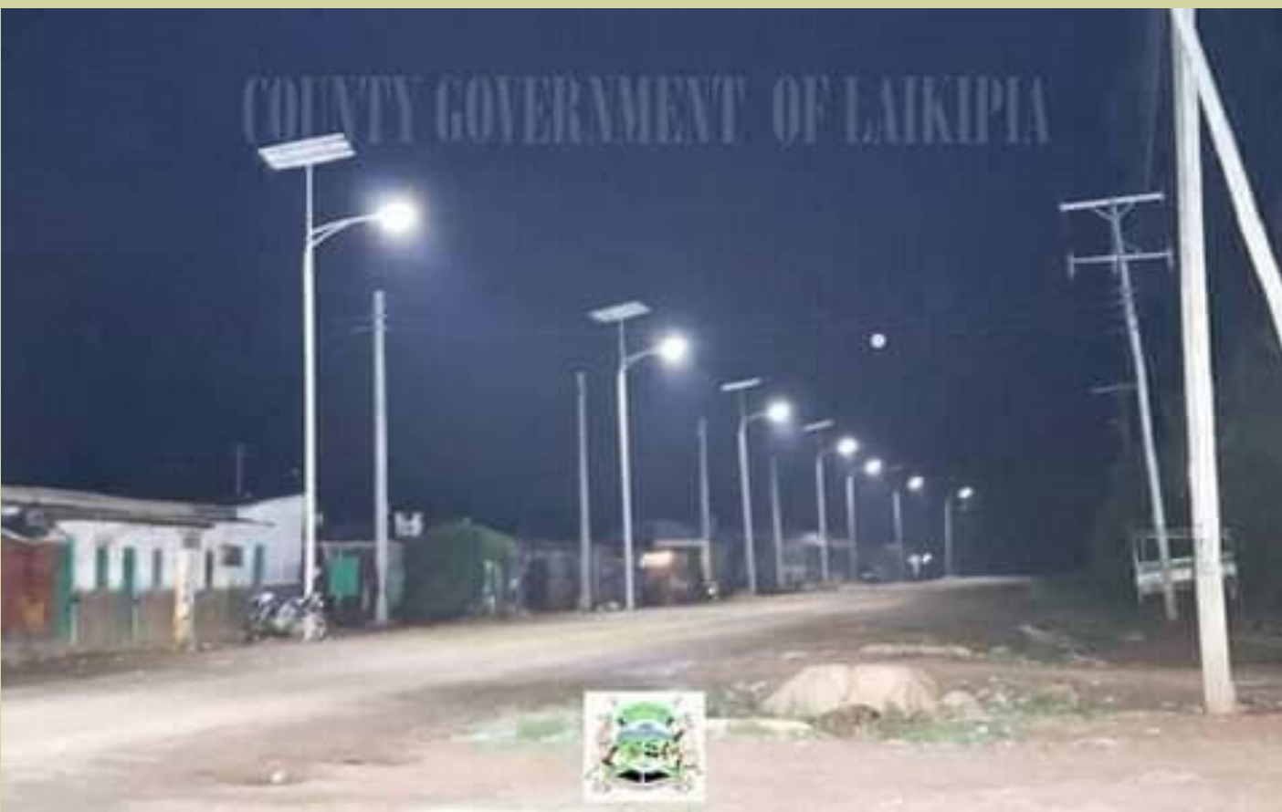
Solar-powered street lights installed at Karaba Market in Marmaent ward under Laikipia smart towns initiative
