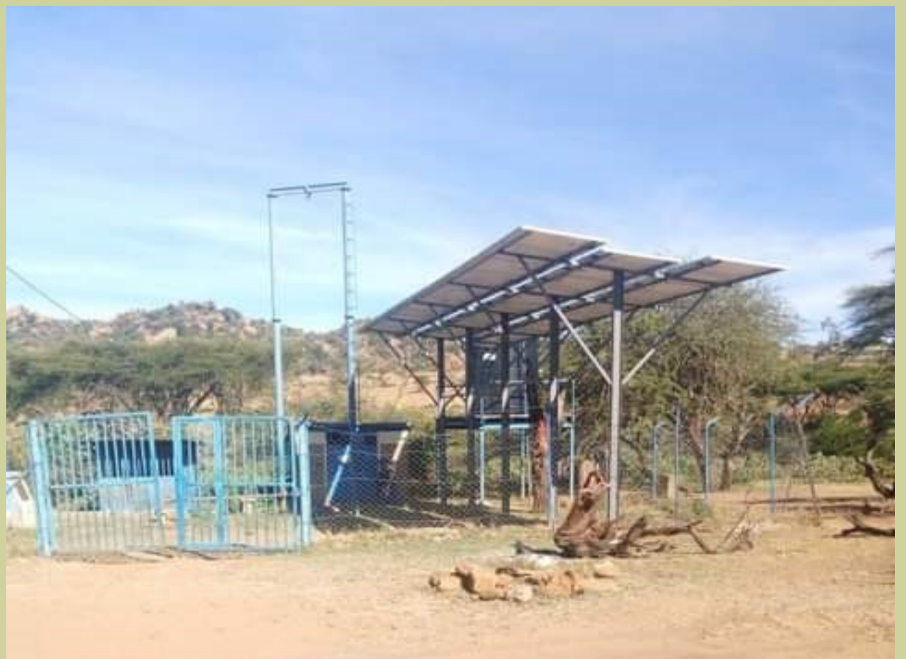
A solar powered borehole in Doldol, one of the many such projects using clean and renewable solar energy to avail water cost effectively
