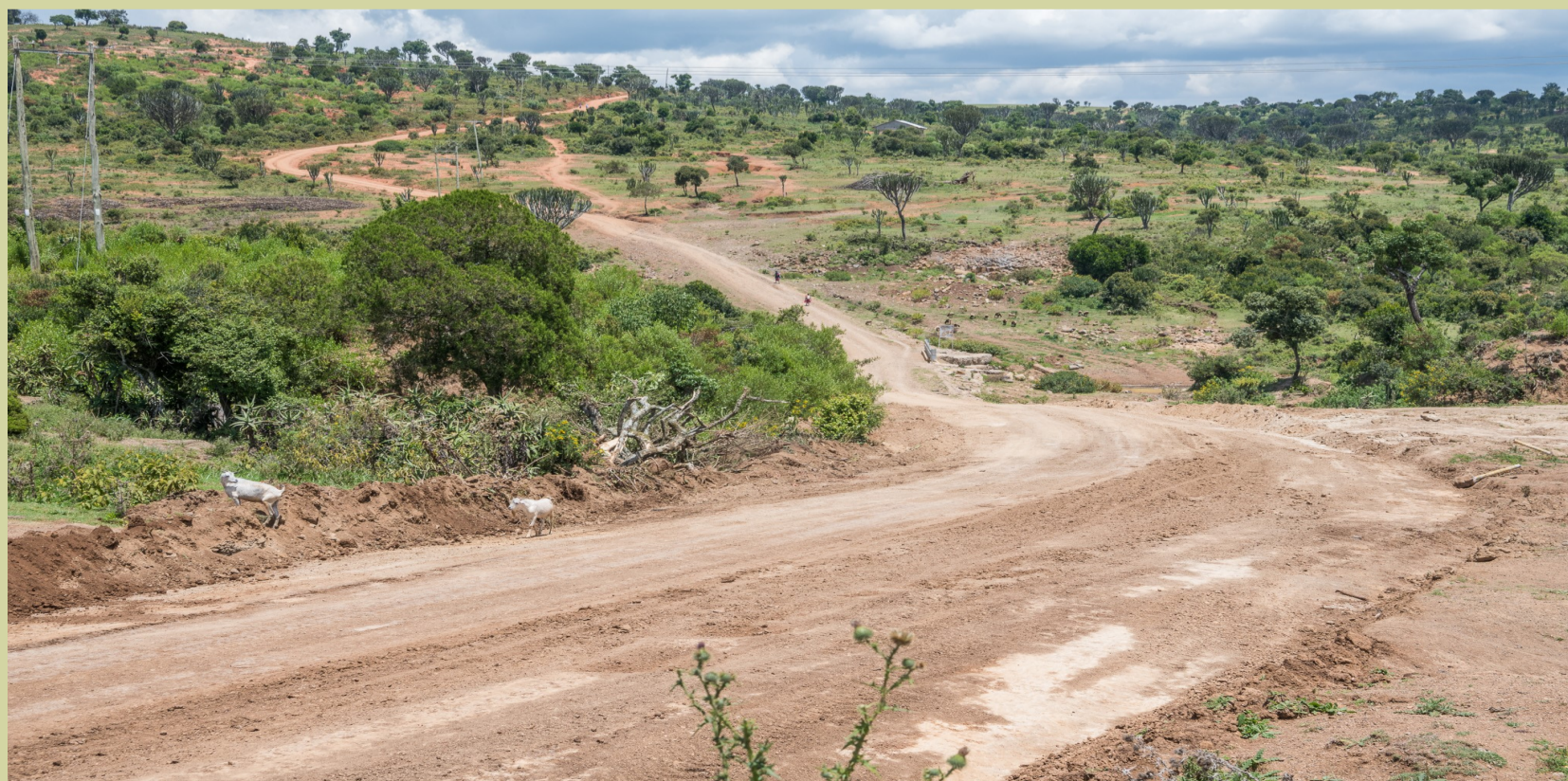
The Chumvi-Arjiju Road which cuts through the scenic Mukogodo Hills Forest is under construction by NYS. The road will link a large section of Mukogodo East ward to Doldol town and promote tourism
