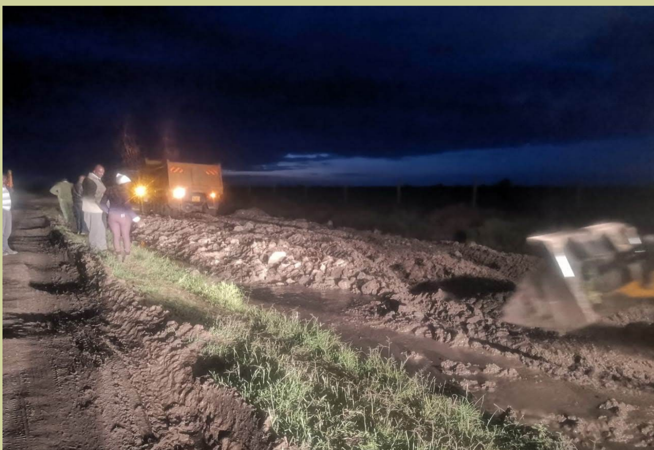
A NEW CULTURE: November 2019 Infrastructure Department workers went out of their way to work overnight to repair the Nanyuki-Rumuruti Road at the Ol Pejeta Gate. Heavy rains had destroyed the road cutting off communication.
