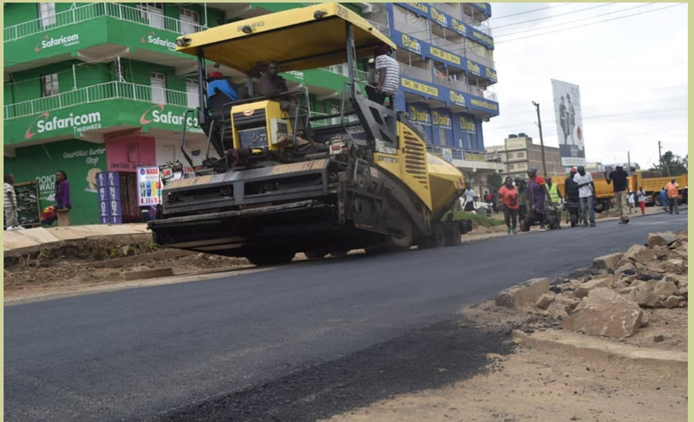
Construction of a road in one of Laikipia's urban centres. Such development are stimulating growth of the county and attracting new investment
