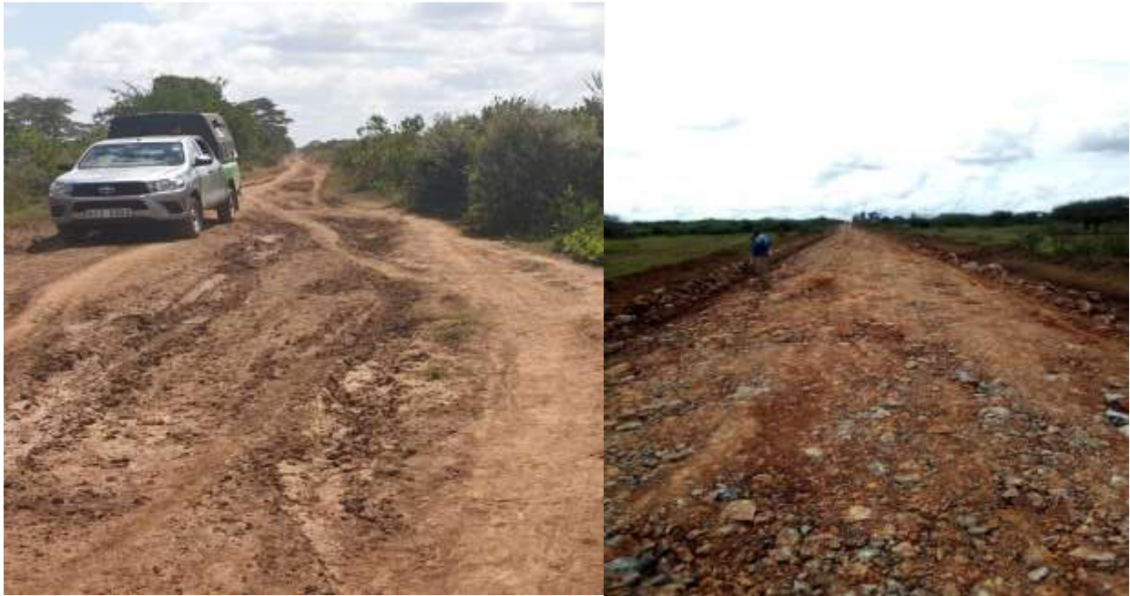
Road improvement under leasing program- Ol Moran Catholic - Kuki Galmann road (before and after)- Olmoran ward
