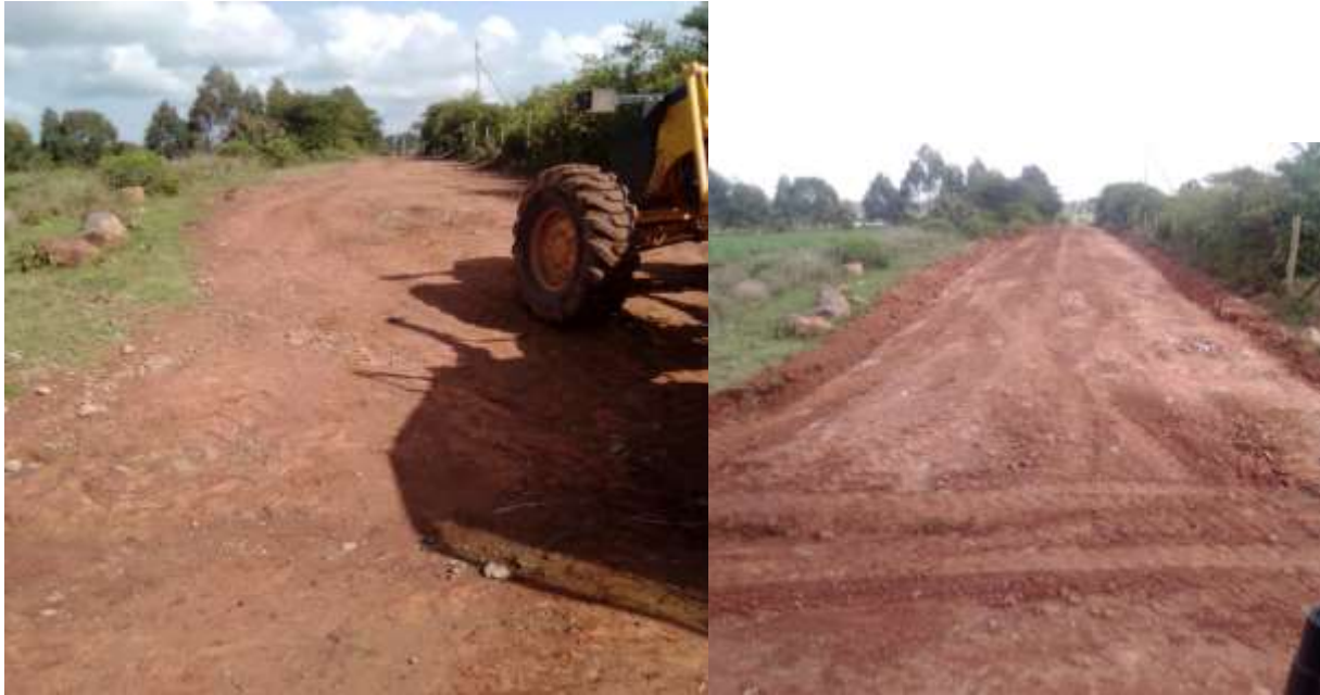
Road improvement under leasing program- Before and After Kahuhu Primary Road-Githiga ward
